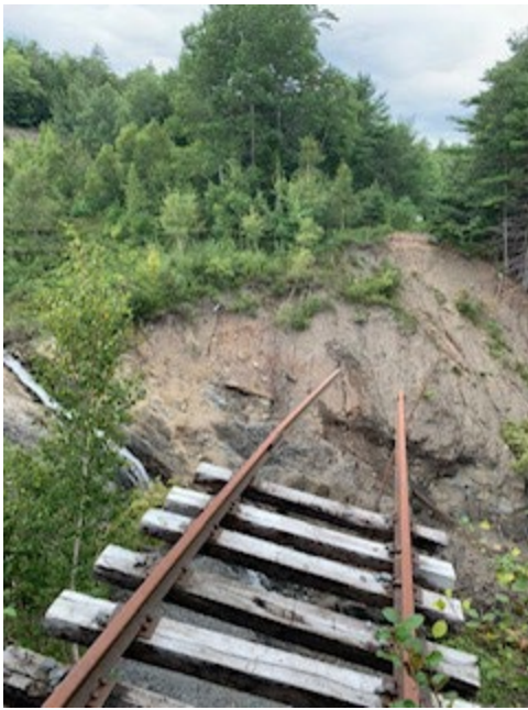
Landslide and washout under the existing windmill closest to highway 101- currently being investigated by the dept of environment.
