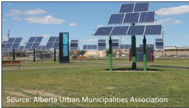
Figure 15: Solar Park in Vulcan, Alberta
